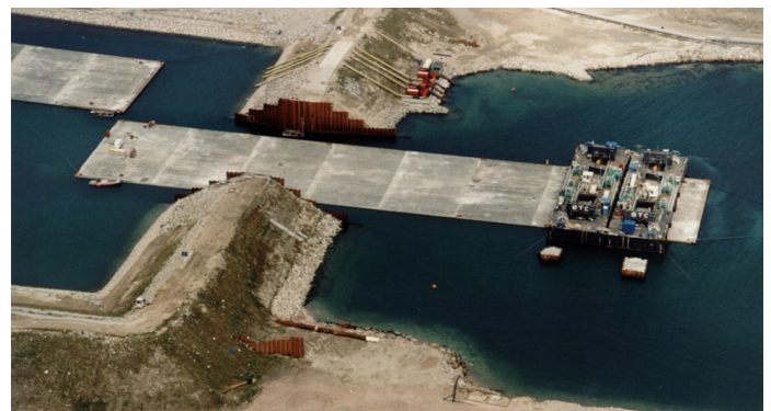
Tow out of completed 176 m long completed tunnel element from casting yard
