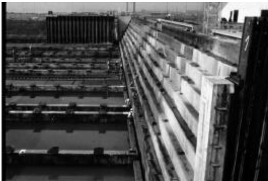
Figure 13 Sliding gate closed, view of the water tight steel skin from basin side
