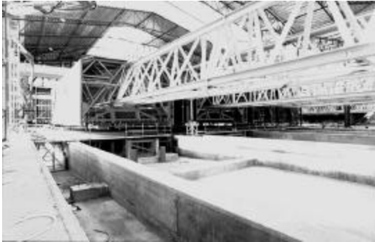
Figure 7 Tunnel form launch girder and, in the background, collapsible bottom forms and movable tunnel shutter
