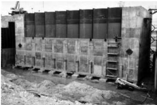
Figure 15 Floating gate match plant cast in the dry on its foundation – sea side view
