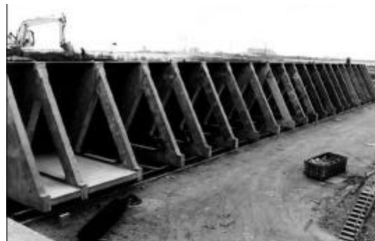
Figure 12 Sliding gate parked in open position view from factory side
