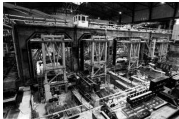
Figure 8 Global view of casting bed – tunnel element waiting to be pushed, two hydraulic rams already in place
