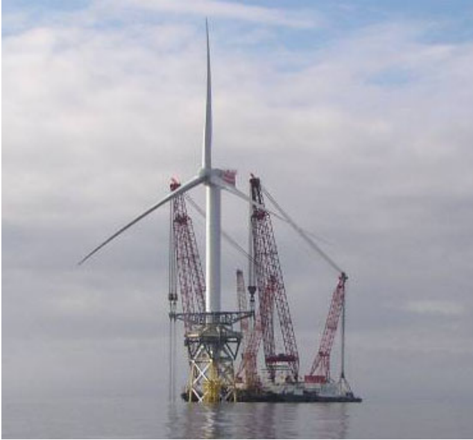
FIGURE 6 INSTALLATION OF REPOWER 5MW TURBINE FOR THE BEATRICE WINDFARM DEMONSTRATOR PROJECT, SCOTLAND
